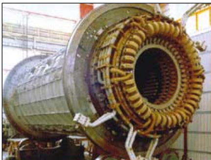
Stator core and winding of a 1000MW generator.
