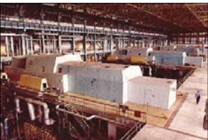
The machine hall of Tusimice Power Station in the Czech Republic, showing the four 200MW units.
