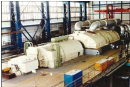
The 500MW steam turbine generator at Melnik Power Station in the Czech Republic.
