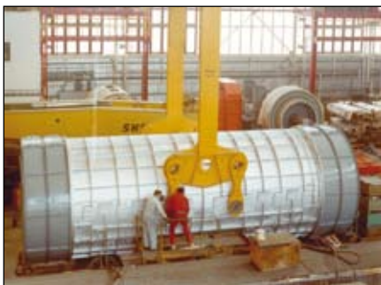
The unrolled stator core of a 1000MW generator.
