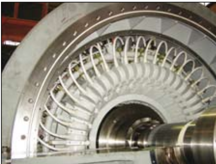
The stator endwinding of a 500MW generator, showing the PTFE hoses that supply the cooling water.
