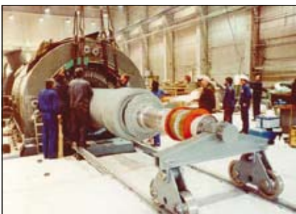
Inserting the rotor of a turbogenerator at Sevo Power Station in Finland.
