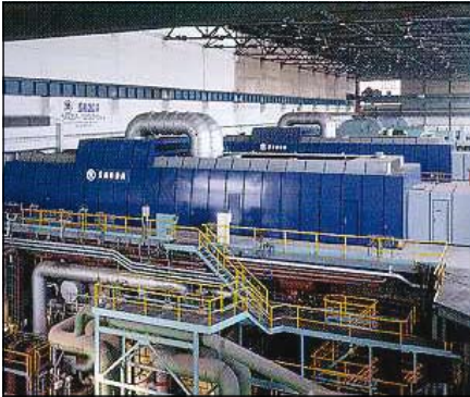
The machine hall of Melnik II Power Station in the Czech Republic.
