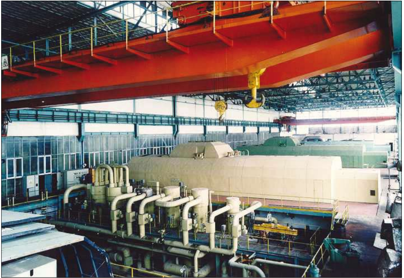
The machine hall at Vojan Power Station in the Slovak Republic.
