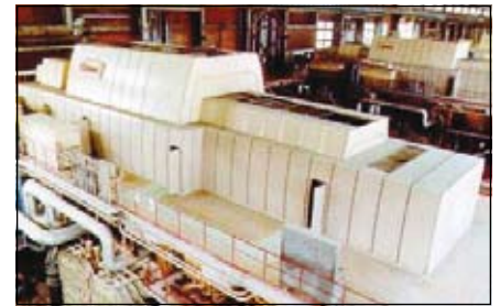
The machine hall of Soma Power Station in Turkey.
