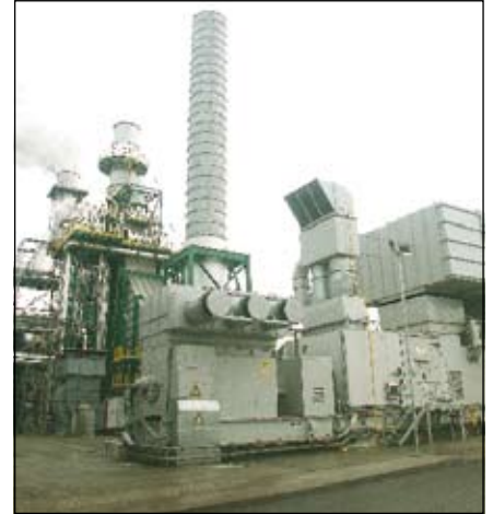
26MW generator with closed circuit cooling air-to-air) at a cogeneration plant in Spain.
