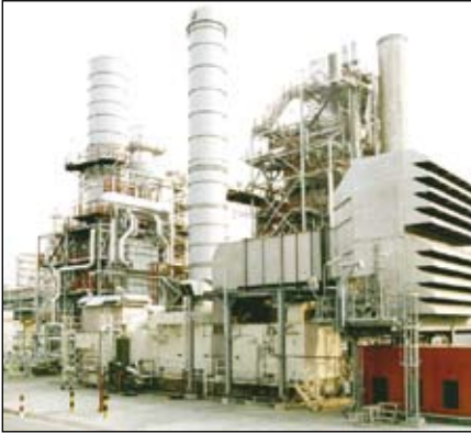
21MW gas turbine driven generator with a multi-stage air inlet filter system.
