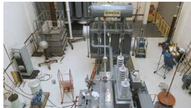
VBO transformer at High Voltage test bay
